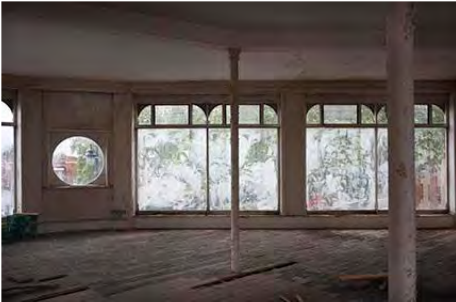
Figure 51 Inside the corner building on the second floor. The circular window originally held a clock.
